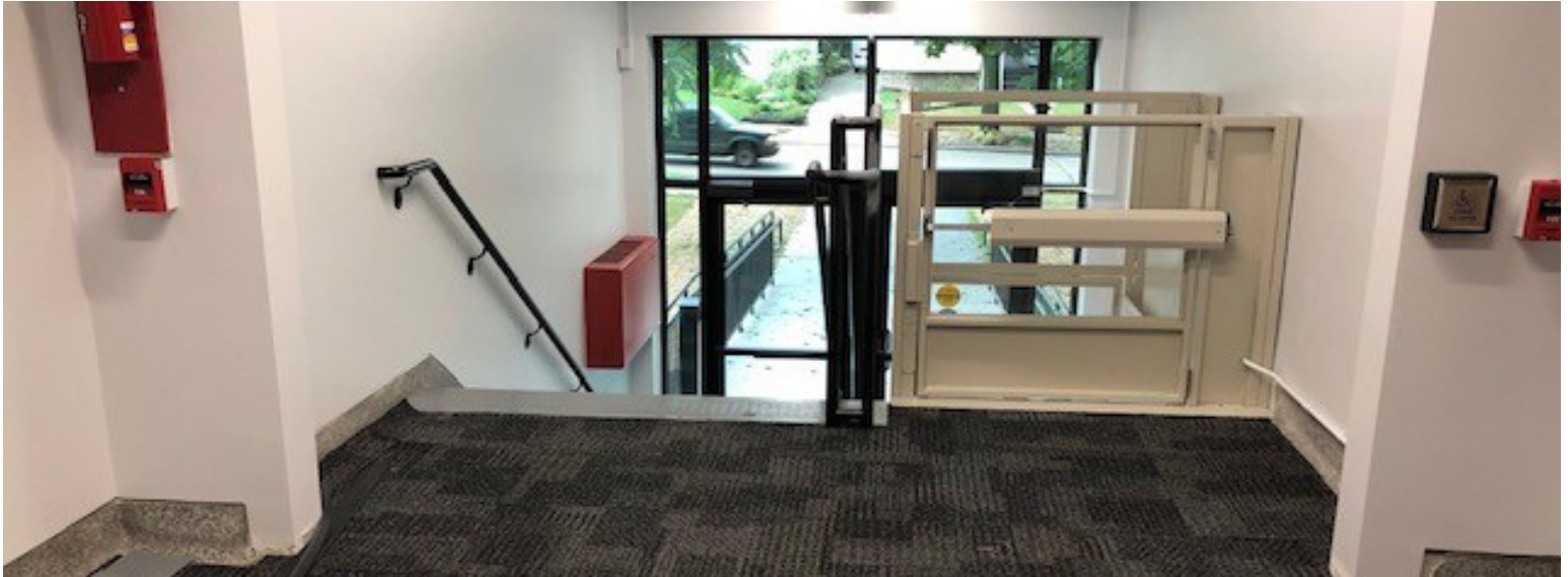
Lift in Main Entrance
