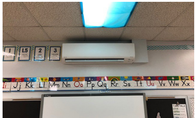
Split Unit in Classroom
